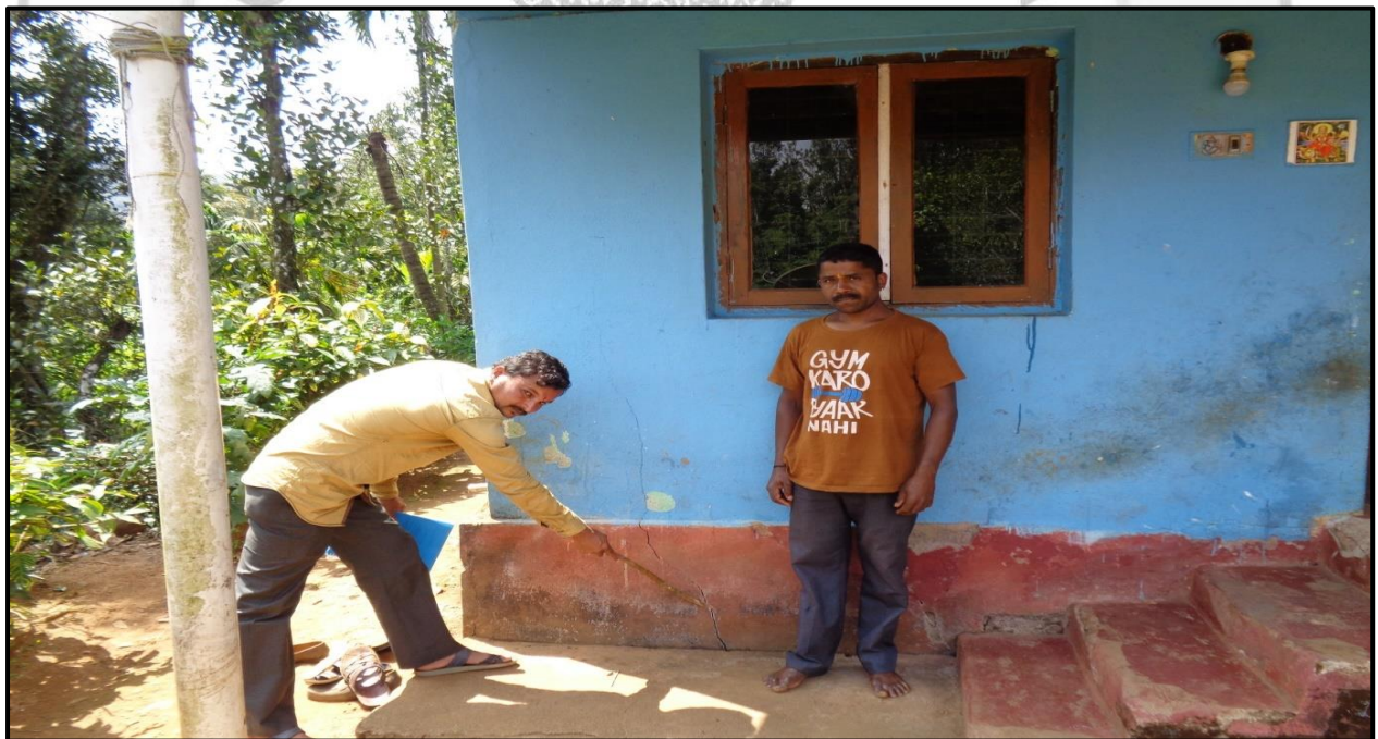
Photo 5: Cracks affected house near Bomarakallu homestay.
