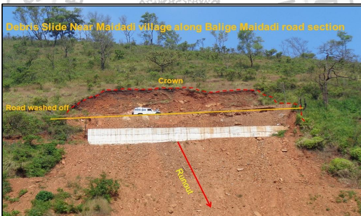
Photo 4: Major treated landslide near Maidadi estate
